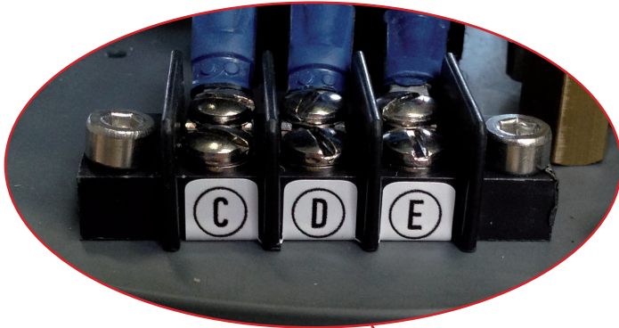
connection at 3-way valve
